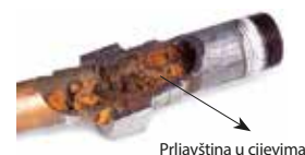
Filter u kotlovnici
